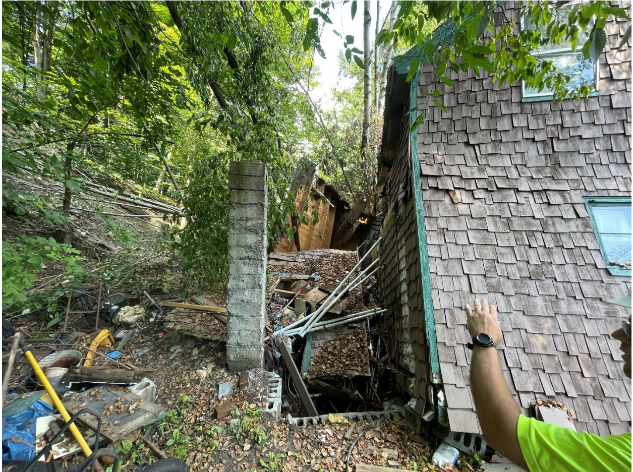
Photograph 1: Close-up view of the house at 5 Portland Street, Barre, Vermont showing approximately 6 feet of displacement from the block foundation. Photograph taken August 4, 2023.
