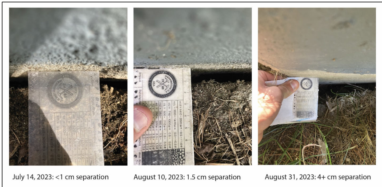
Photograph 2: Separation of the soils from the foundation at the northwest corner of the house. The separation opened up during the July 10-11 storms but did not widen significantly for the ensuing month, but then significantly widened between August 10-August 31.
